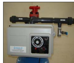
Fleck 2750 with PVC pipe work
